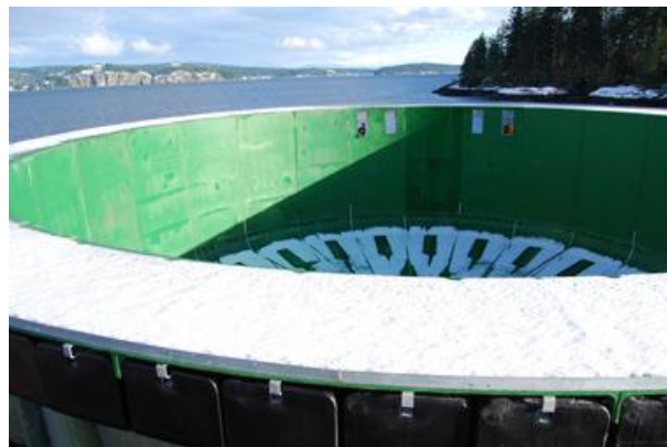
Eric Joseph, top centre, is dwarfed by the new closed-containment tank built at Middle Bay north of Campbell River as he works on one of the massive tank's overflow ports. The Middle Bay Sustainable Aquaculture Institute and partners Agrimarine Industries hope to have 50,000 young chinook salmon swimming in the tank within two weeks. Quadra Island can be seen in the distance.
